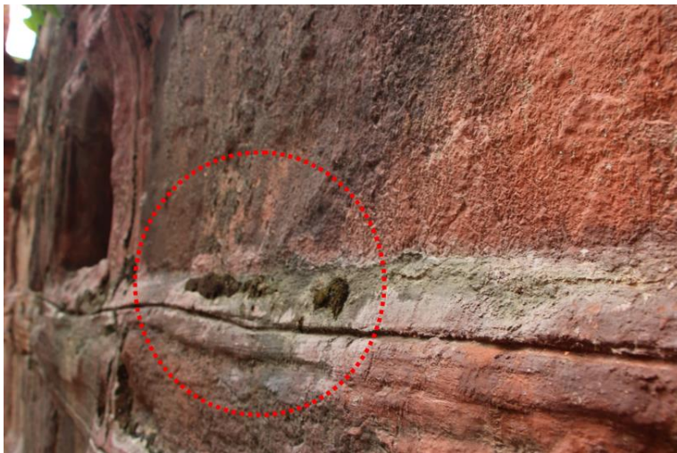
Figure 10: Change in physical and chemical properties of stone
